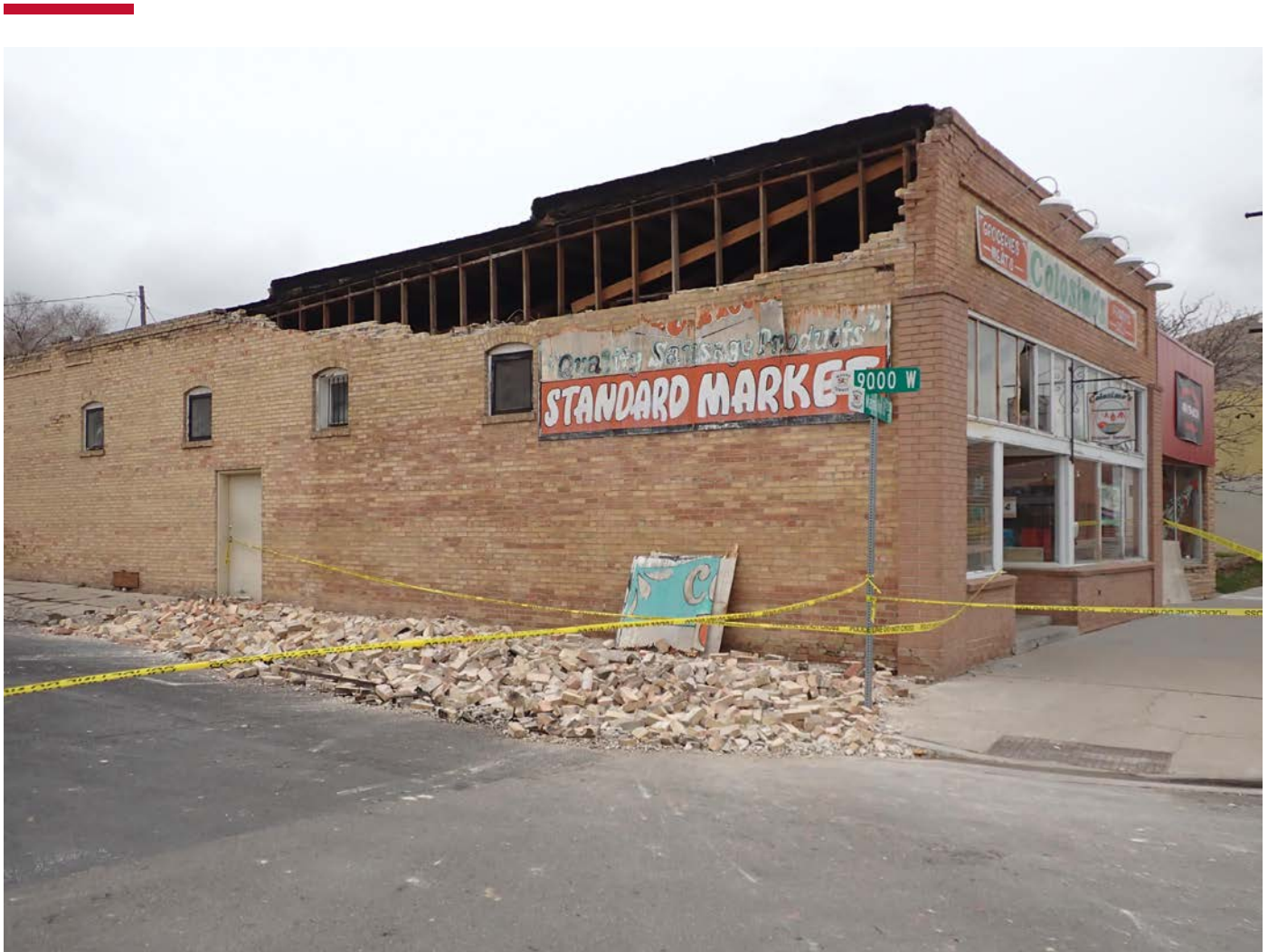
FIGURE 5: Particularly vulnerable to seismic events, unreinforced masonry buildings are often prioritized in retrofit programs.
