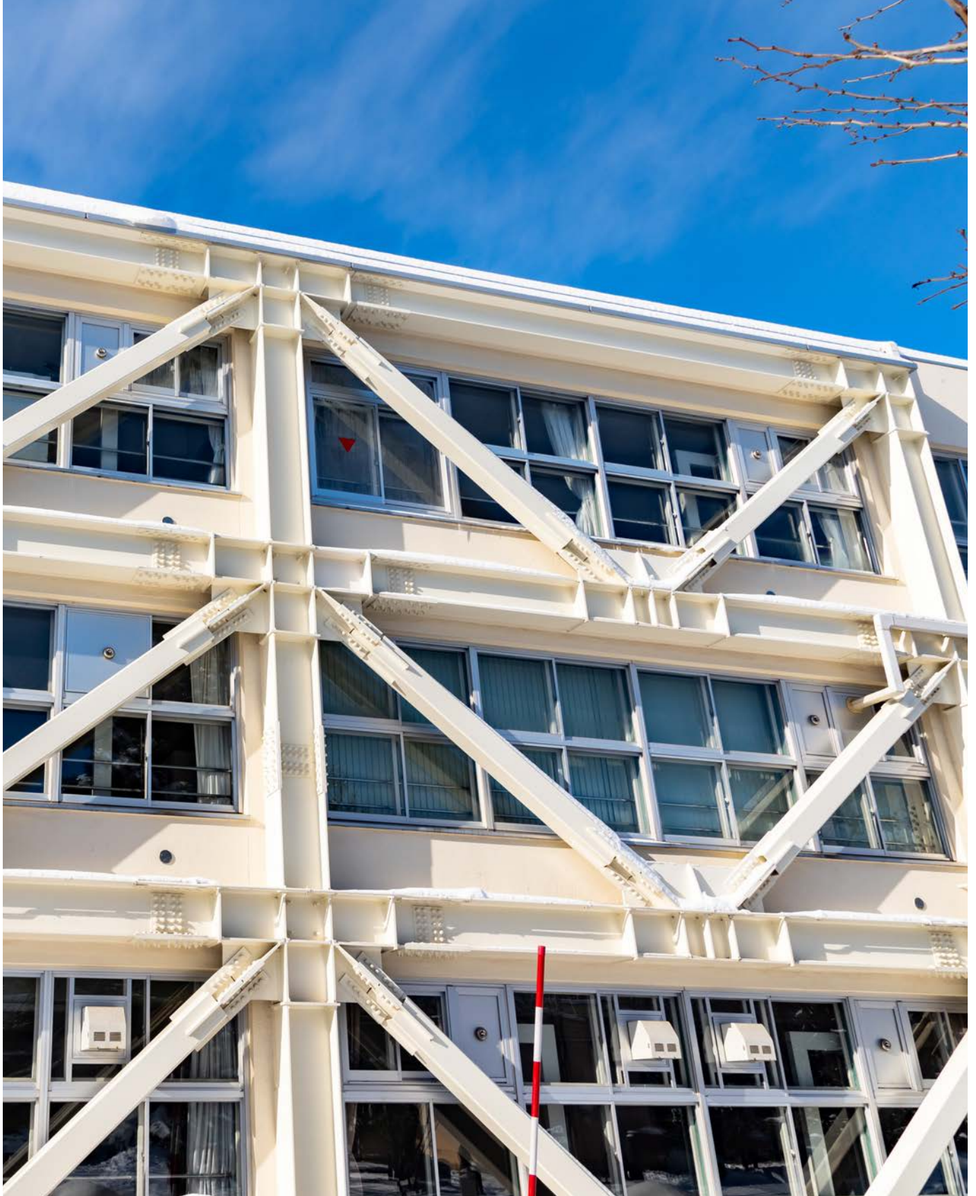
FIGURE 1. Retrofit programs can help the wider community.
